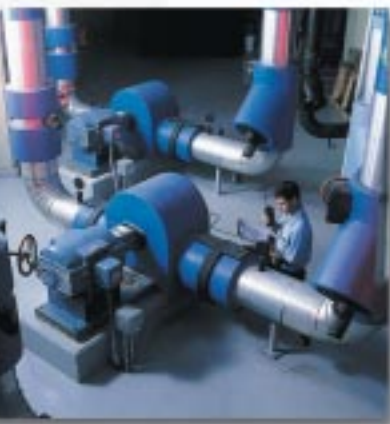
Traditional pump room application for VFDs
